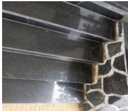
Figure 6. Floor Cracks in the Auditorium Building of the Defense University
