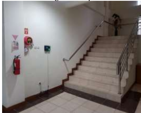
Figure 7. Fire Extinguisher in the Dean's Building of the Faculty of National Security, University of Defense
