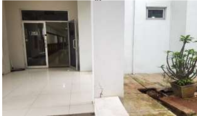
Figure 4. Cracks in the Columns of the Defense University Auditorium Building
