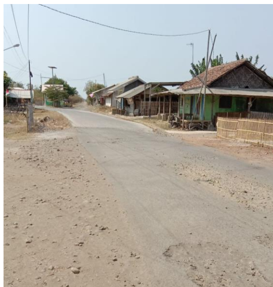
Picture 1. Damaged, sandy, rocky, and potholed Cantigi Road
